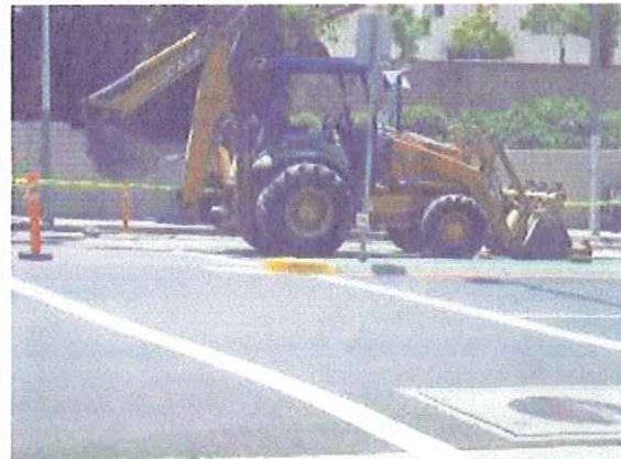
This was taken after the "SIDEWALK CLOSED" signs were in place. The stanchion posts and caution tape were not in place on the northside of the trench.
