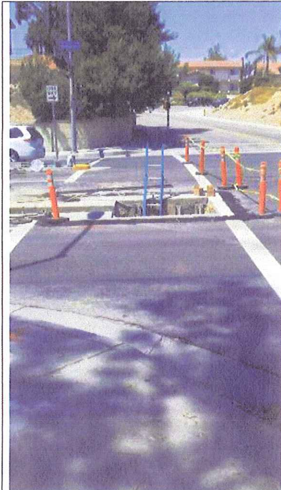
This was taken the day of the risk assessment. The crosswalk was open and there was no protection across the trench openings.
