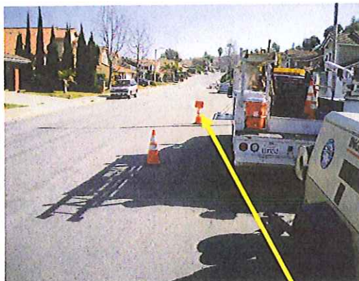
End construction sign too close.
